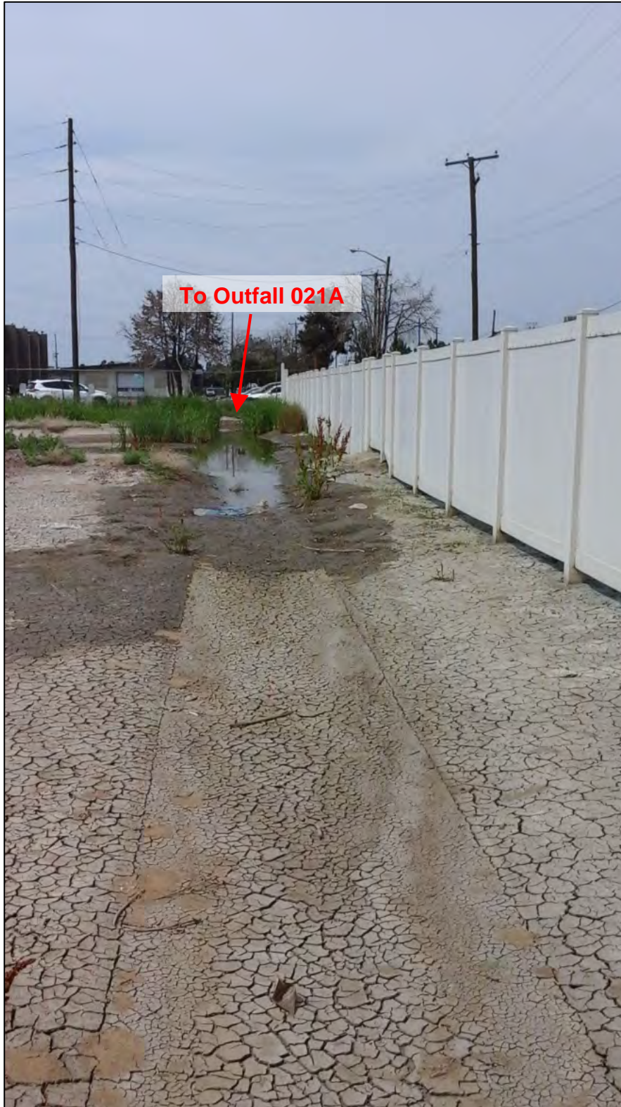
Photograph 15. View, facing north, of a valley gutter leading into the stormwater detention basin shown in Photograph 14. Note the accumulated sediment in and around the valley gutter.
