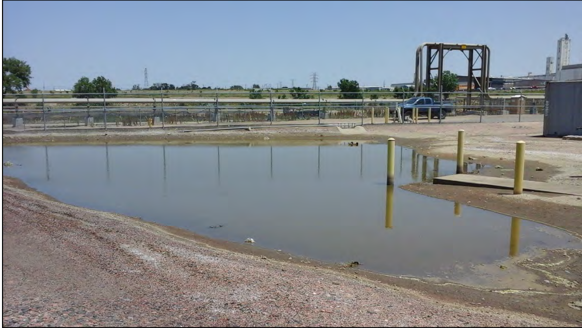
Photograph 11. View, facing northeast, of the stormwater detention area located immediately east of the GWTS. This stormwater detention area overflows towards the Sand Creek Swale Pond and to the stormwater detention area before discharges to Outfall 023A. This stormwater detention area is not identified in the SWMP.
