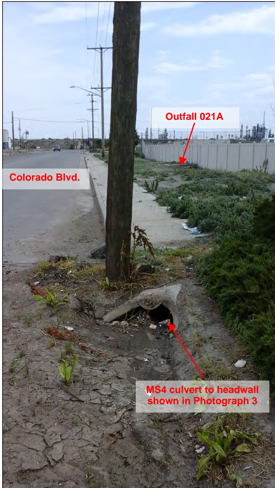
Photograph 4. View of a storm drain culvert inlet along Colorado Boulevard adjacent to the Nelson Property. This MS4 culvert outlets at the headwall shown in Photograph 3 at the same location as Outfall 021A from the Nelson Property.
