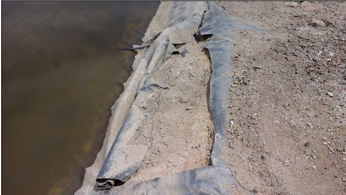
Photograph 36. Close-up view of the torn poly liner of Webber's Pond shown in Photograph 33.
