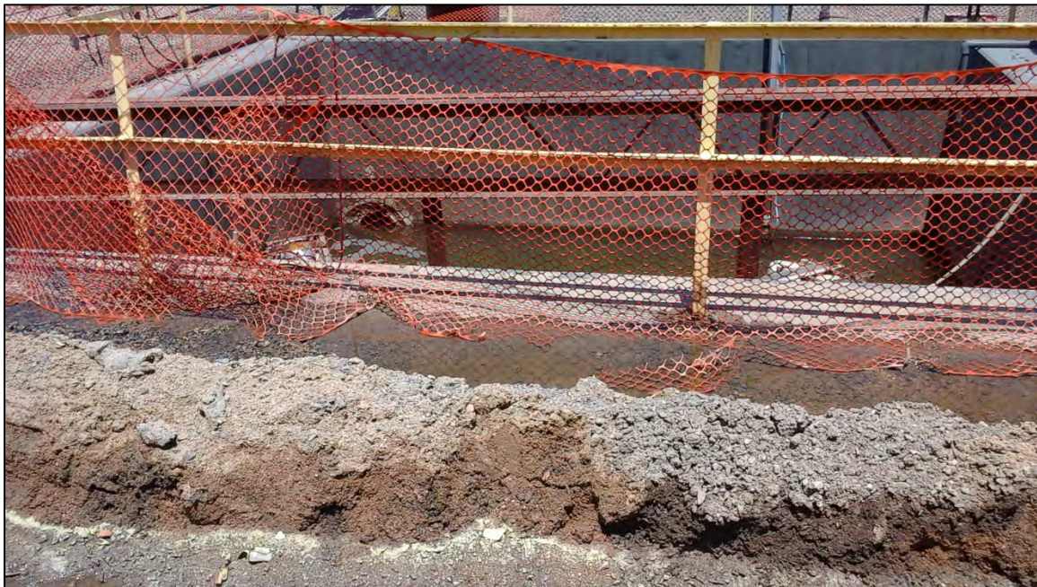
Photograph 8. Additional view of the unconsolidated sediment and gravel berm upgradient of Outfall 020A aerated sampling vault, as shown in Photograph 7.
