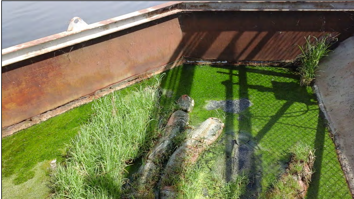
Photograph 13. View of accumulated solids and vegetative growth in the Lagoon No. 1 forebay which receives flow from the “Morgan Box.”
