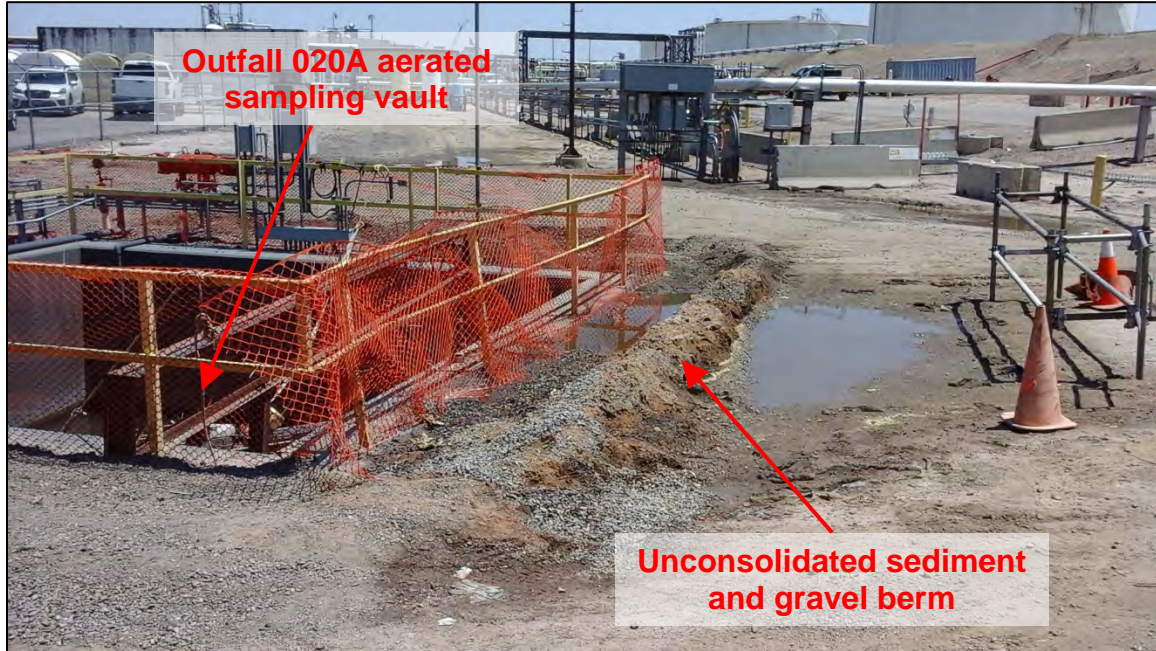
Photograph 7. View, facing east, of an improperly installed (i.e., unconsolidated) sediment and gravel berm located upgradient of the Outfall 020A aerated sampling vault. Note the berm was constructed to prevent contaminated stormwater runoff from Plant 1 from entering the uncovered sampling vault, which had occurred on May 22 and May 31, 2021, resulting in high levels of benzene and BTEX and a visible sheen into Sand Creek. Also note the accumulated stormwater runoff against the berm.
