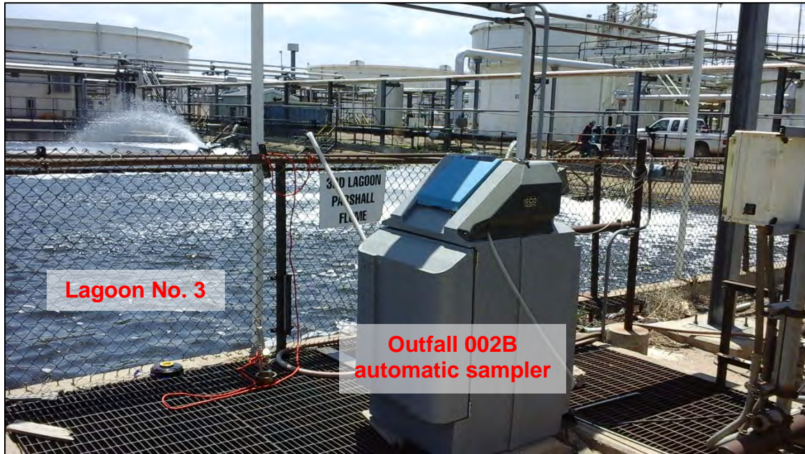
Photograph 5. View of the ISCO 4700 automatic composite sampler at Outfall 002B, downstream of Lagoon No. 3. This sampler was not equipped with an independently calibrated thermometer.
