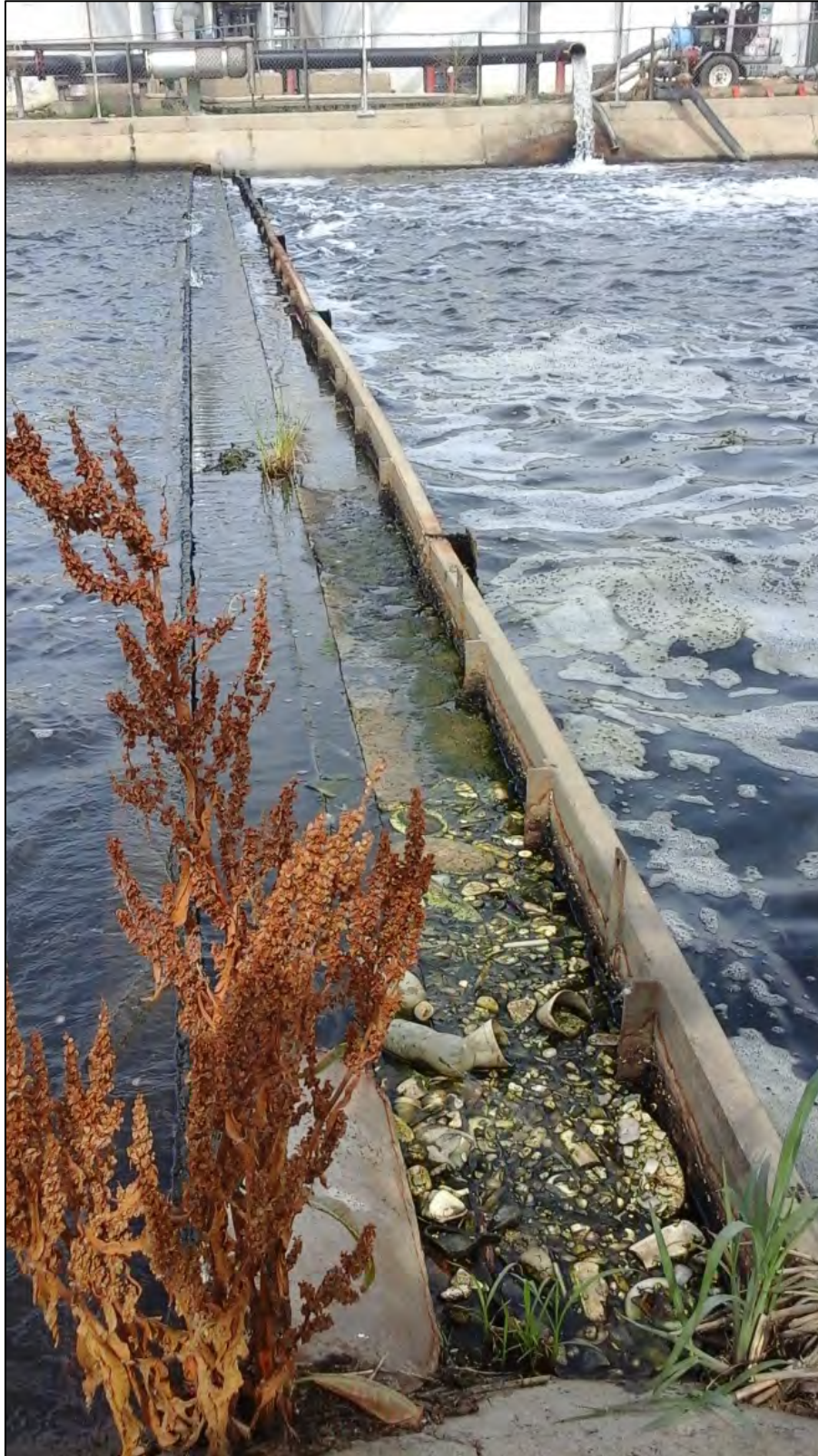
Photograph 12. View accumulated solids and vegetative growth at the weir between Lagoon Nos. 2 and 3.
