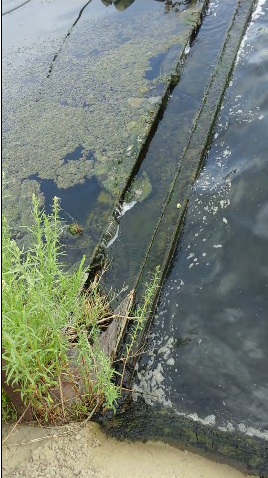
Photograph 11. View of accumulated solids and vegetative growth at the weir between Lagoon Nos. 1 and 2.
