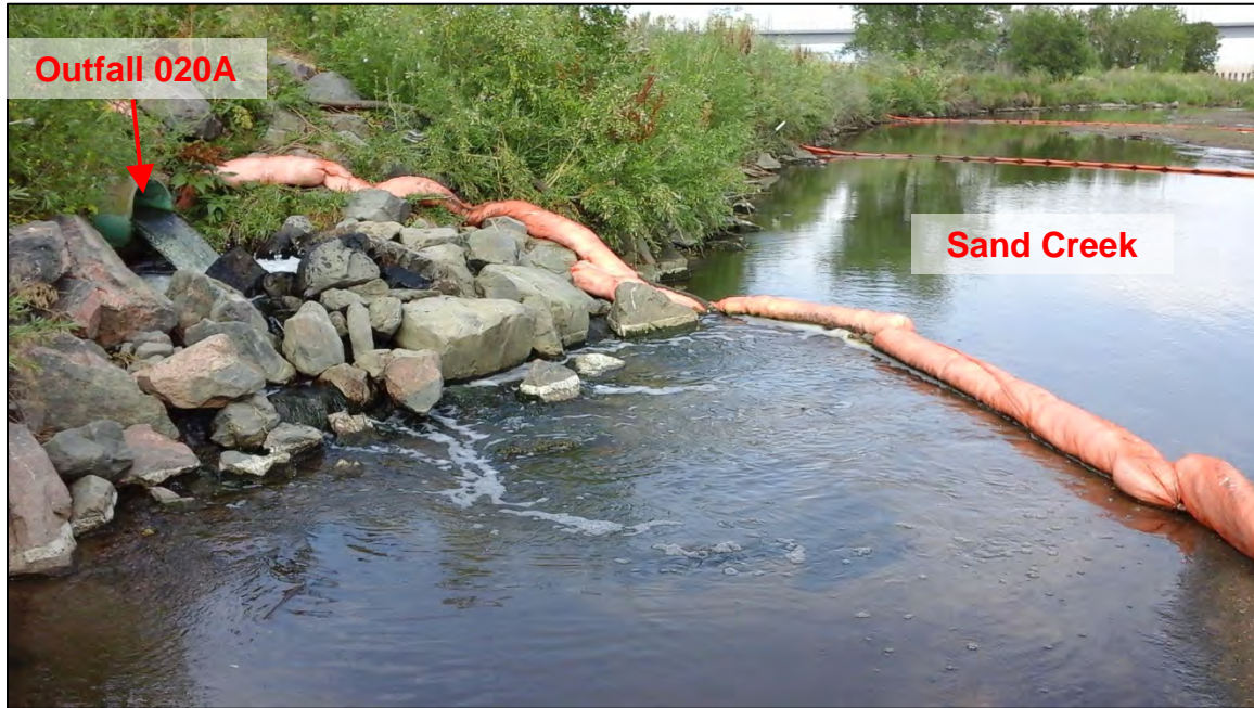
Photograph 1. View of Outfall 020A to Sand Creek.
